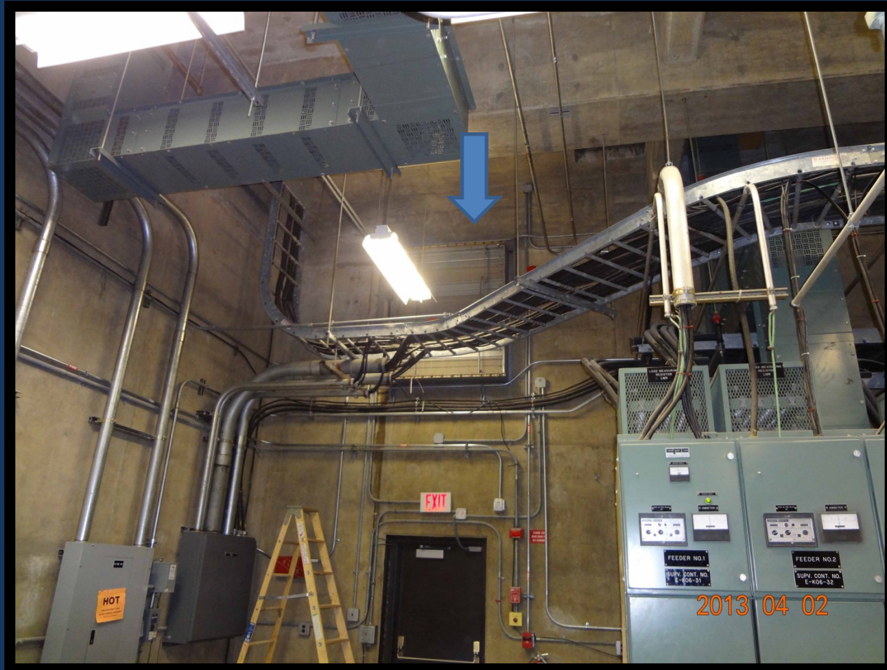
Existing motorized dampers to be replaced
