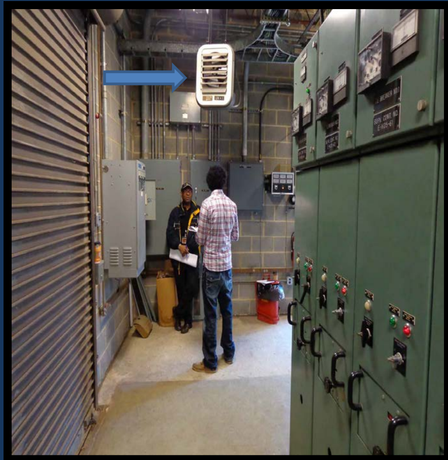
Existing unit heater to be replaced
