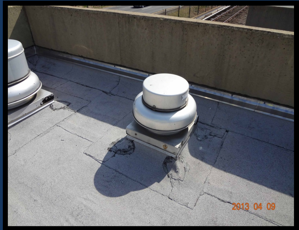
Existing battery exhaust fan to be replaced
