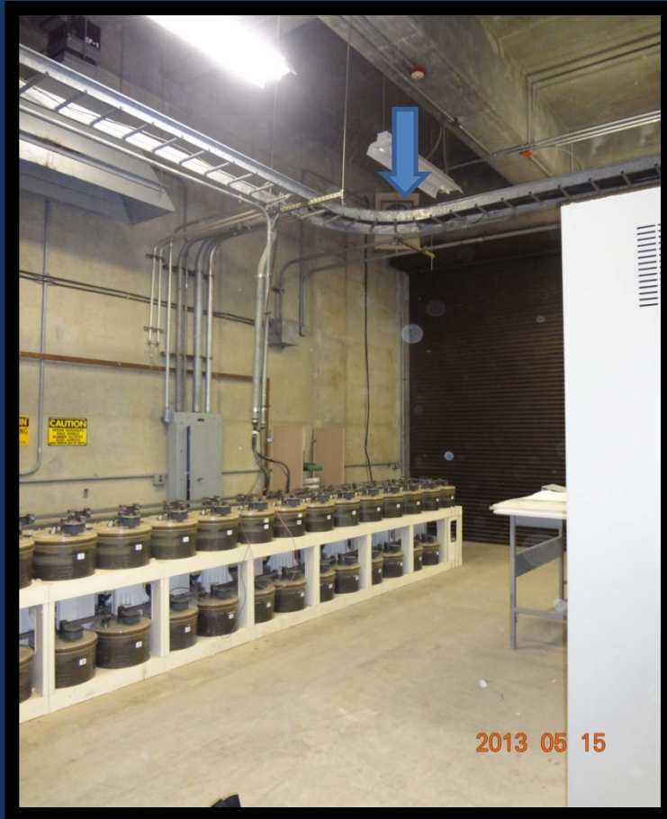
Existing heater to be removed/replaced
