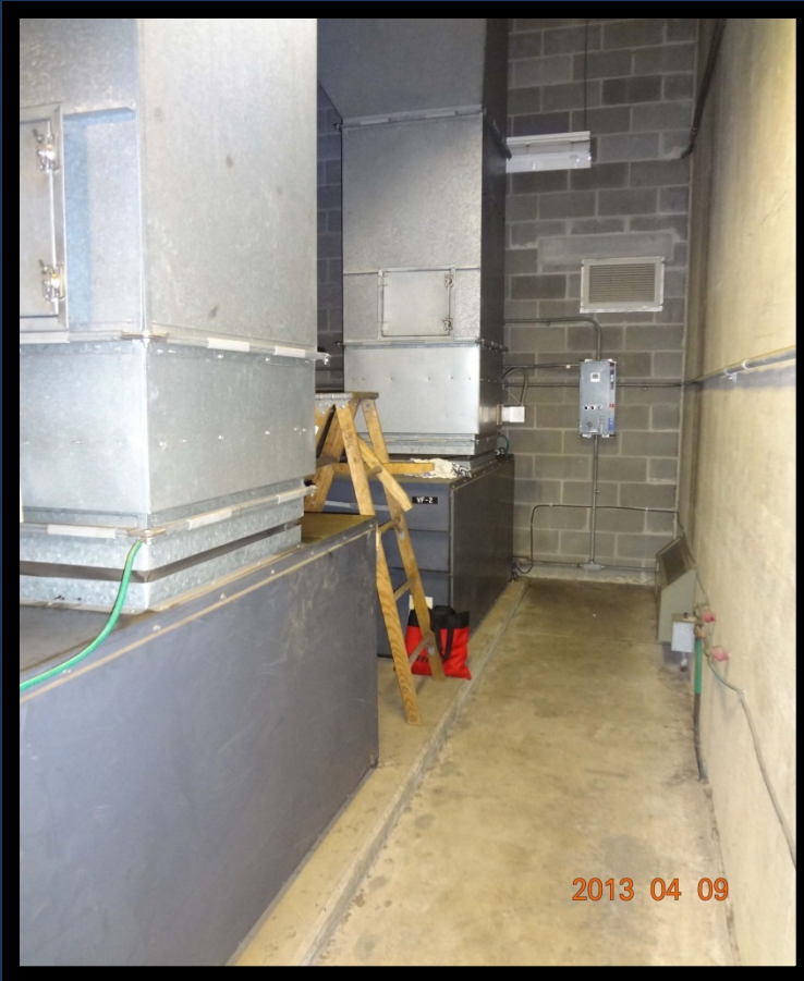
Existing supply fans to be replaced
